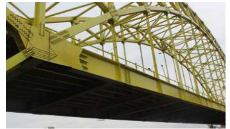
Online Monitoring Jembatan Kamojang (Structural Health Monitoring System/SHMS), Bandung – Jawa Barat, 2016
