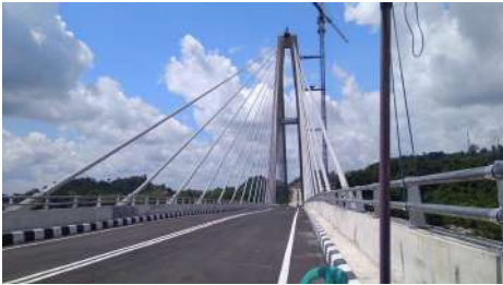
Online Monitoring Jembatan Mahkota II (Structural Health Monitoring System/SHMS), Samarinda – Kalimantan Timur, 2017
