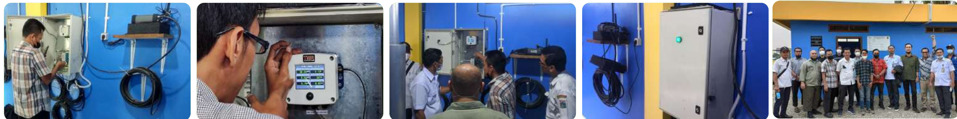
Automatic Water Level Monitoring System - Dinas SDA
